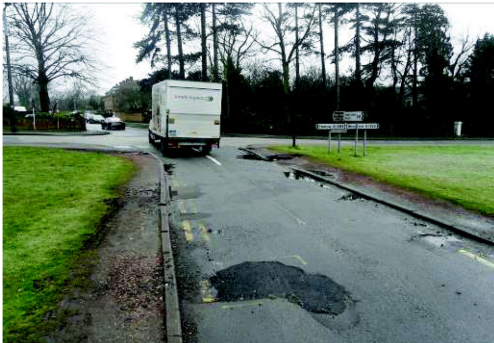
Photo 4 – Link road to the B181 Lindsey Street is in poor condition.
