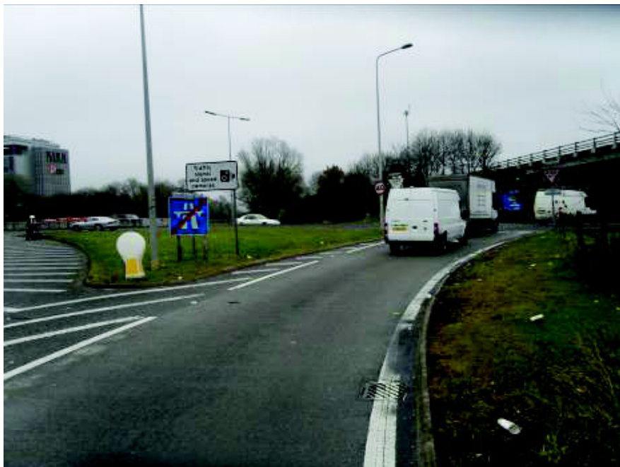
Photo 2 – Sign clutter within traffic island on M11 north-bound off slip.
