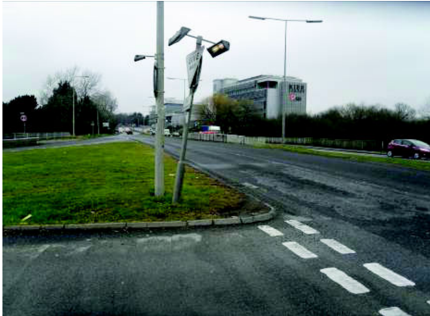
Photo 1 – Nearside 'Give way' sign is partially faded and leaning to one side.
