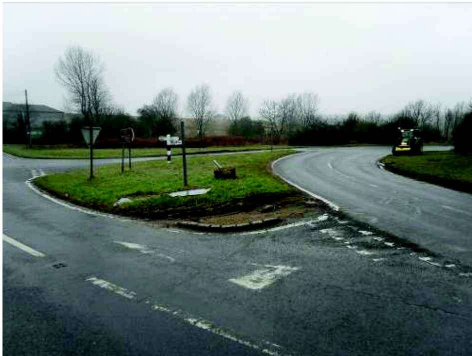
Photo 4 – Worn road markings and damaged / missing traffic signs at junction. Also shows the variations in vertical alignment at the junction.
