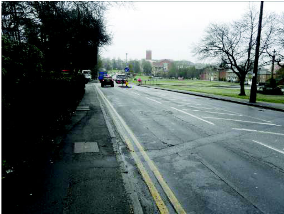
Photo 2 – Narrow footway due to impeding boundary hedge.
